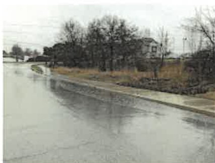
Drendel Road Flooded Street 3.jpg 3990K
