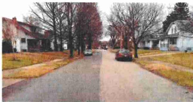
Maltene Rejuvenator: Sustainable Water-Resistant Performance. Image of Ohio roadway years after a maltene rejuvenator was applied and shortly after a rainfall. The treated section is dry, while the untreated section of pavement remains wet
