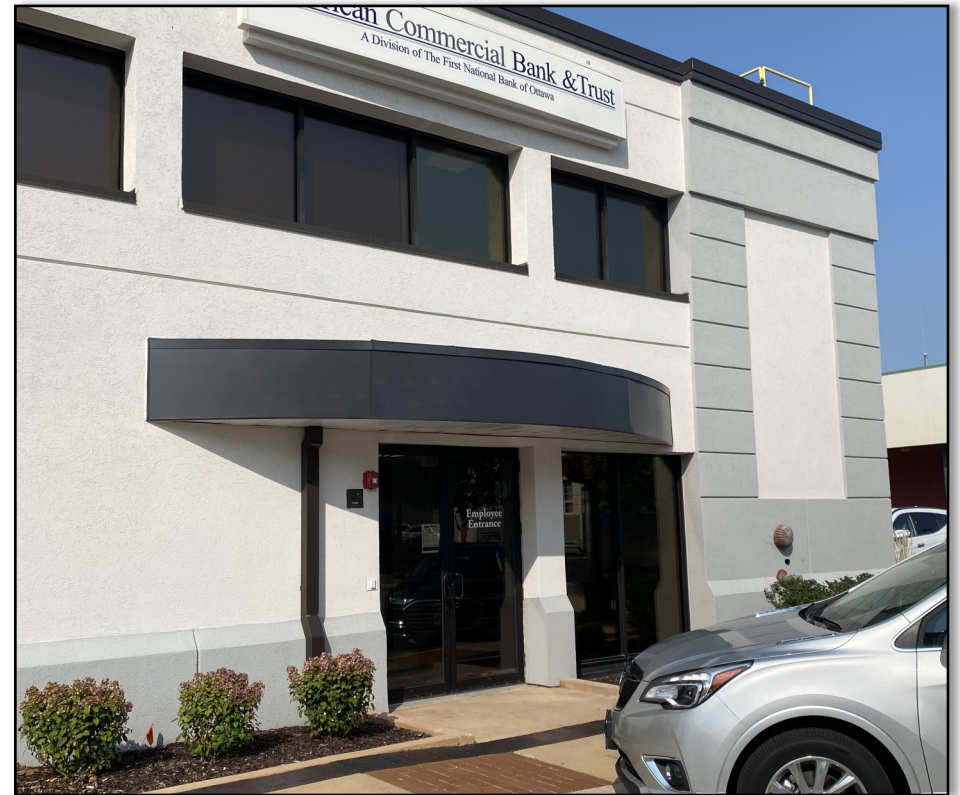
DISCOURAGED — Do not use EIFS as the primary building material.
