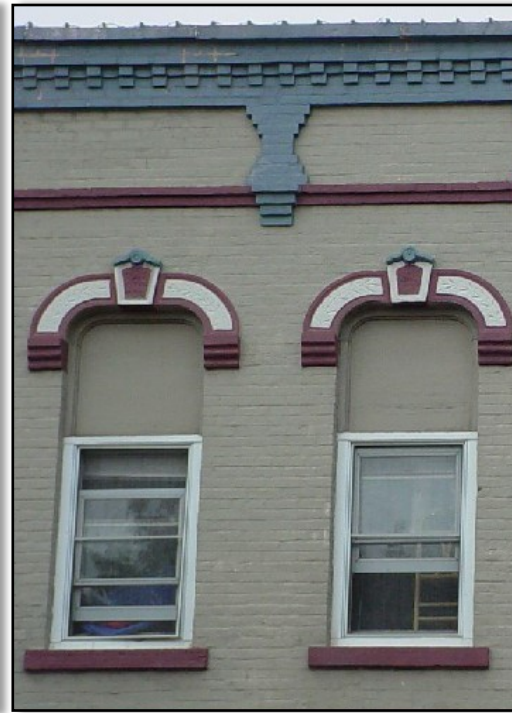
DISCOURAGED — Avoid replacing windows where the window opening is not filled in completely.
