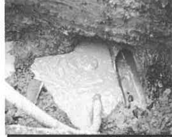
Hidden leak running into drain tile
