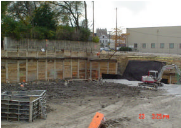
Earth retention system in southwest corner of storm A7 water detention basin.
