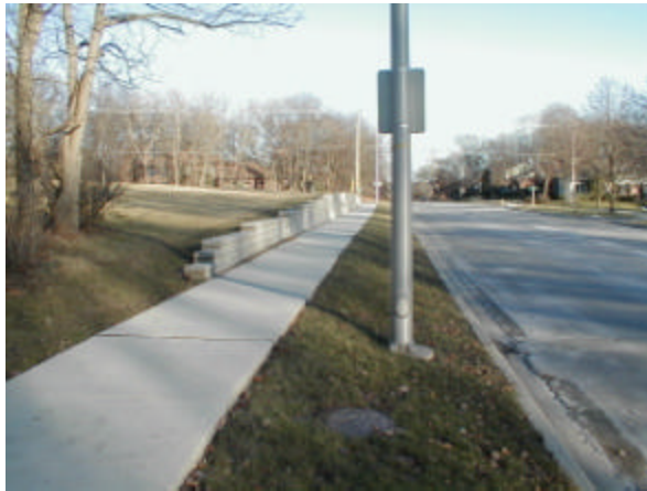
35 th Street as it meets Saratoga Street Retaining wall with steep parkway grade.
