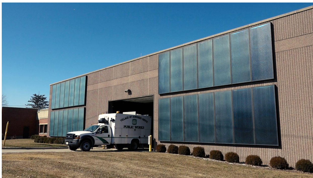
Solar panels on the Public Works building
